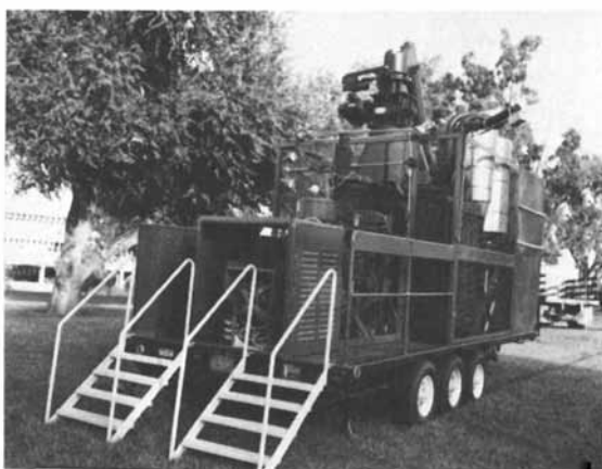
Figure 6. Complete energy conversion system (100 KVA engine-generator is in foreground)
