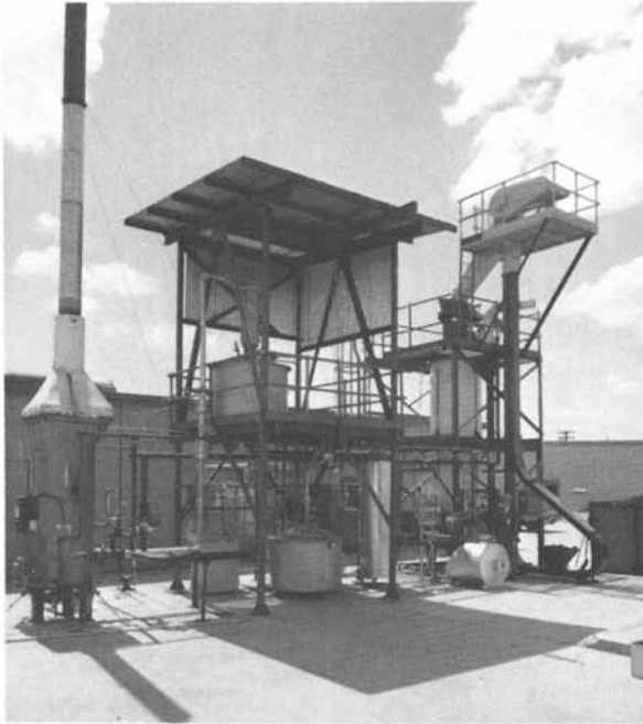
Figure 6. Three-foot gasifier and hot gas clean up pilot plant
